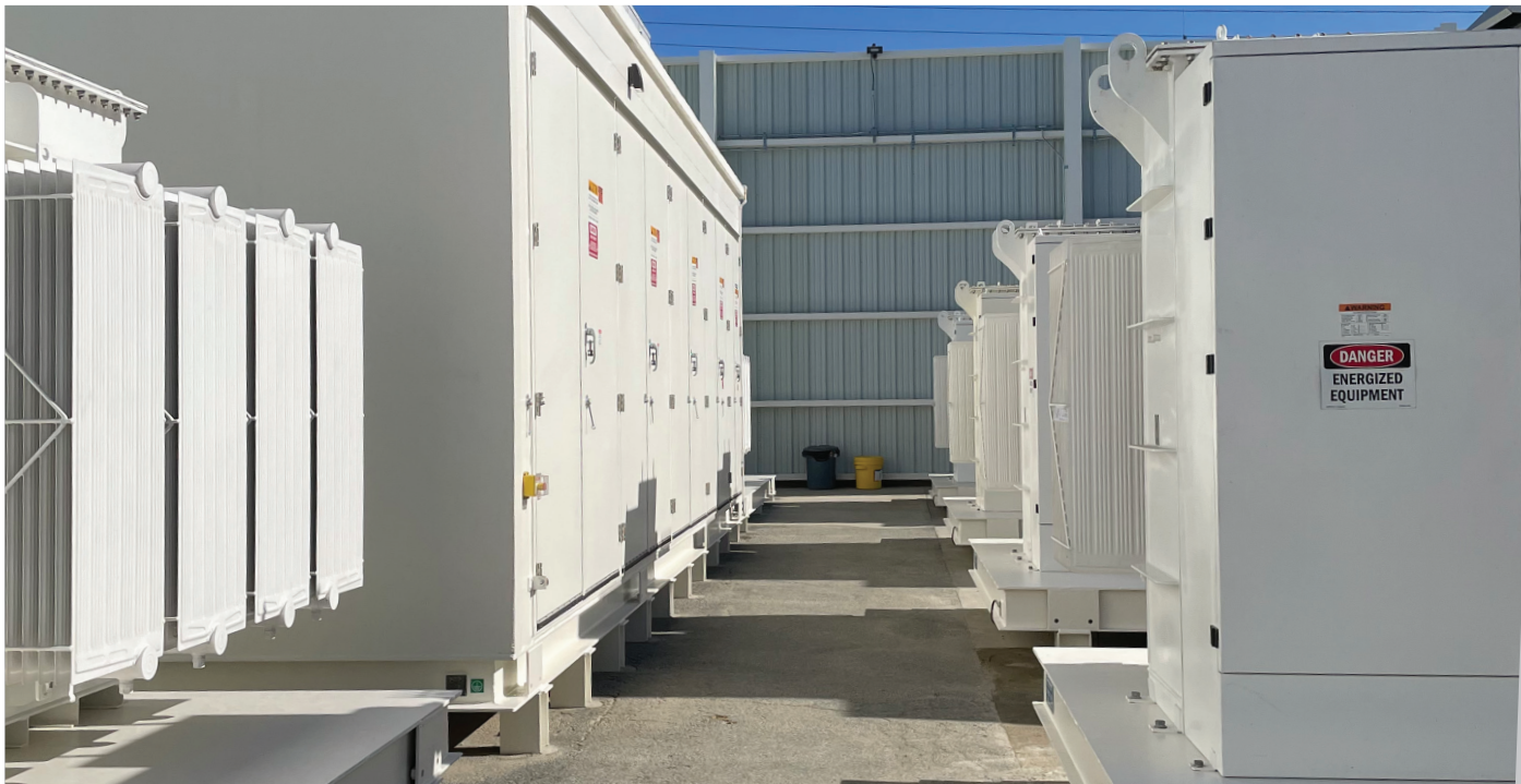
Wellhead Stanton | Energy Vault | Stanton, CA 68.8MW/275.2MWh BESS
