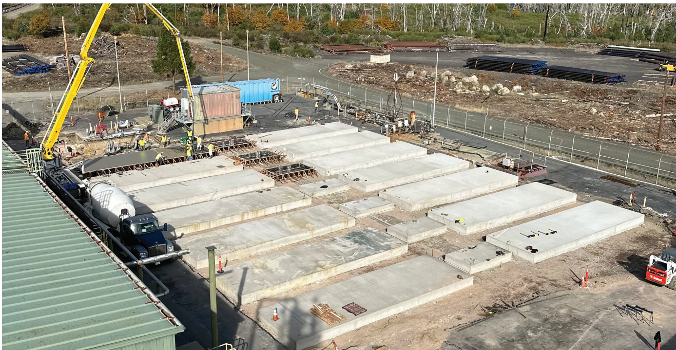
Geysers | Calpine | Middletown, CA 60MW/240MWh (re-purposed thermal plant) BESS
