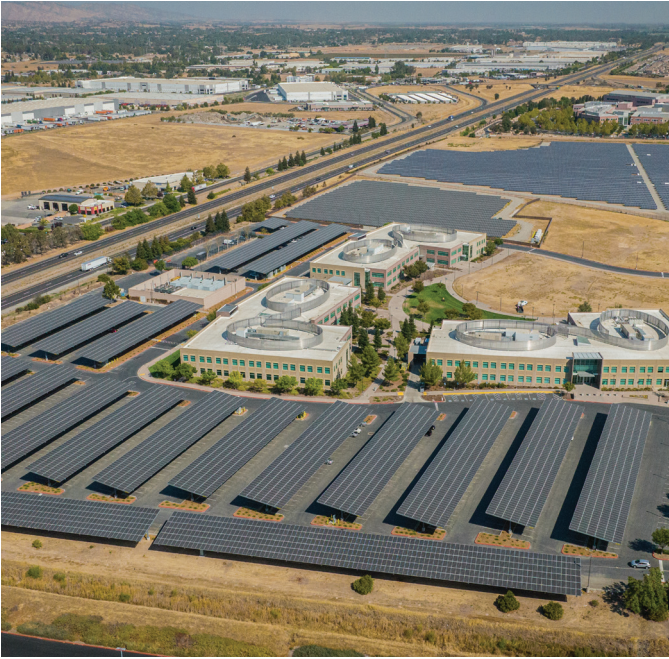
State Fund Portfolio | Vacaville, CA 10.6MW distributed generation (across 4 sites) Vacaville, Pleasanton, Redding, Sacramento Solar | EV Charging | BESS
