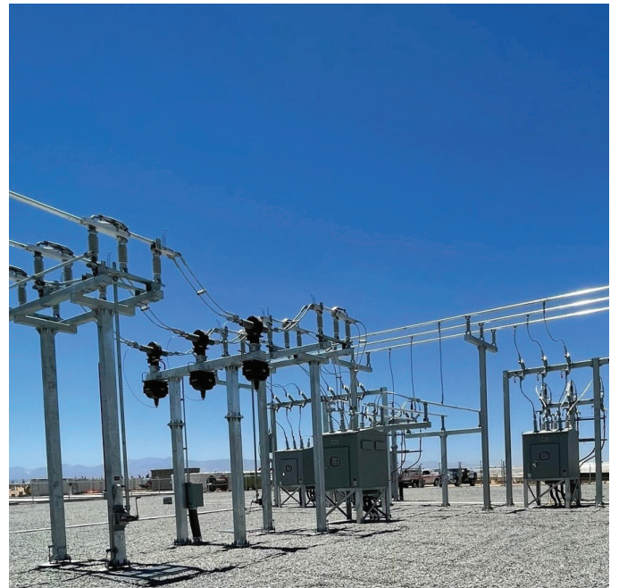
High Desert | SOLV Energy | Victorville, CA 230kV substation Substation
