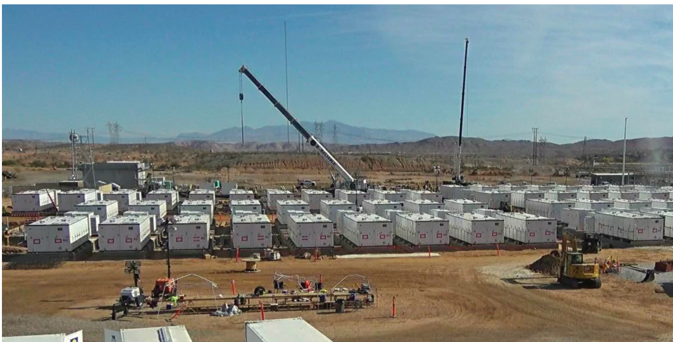
Reid Gardener | Energy Vault | Moapa, NV 220MW BESS
