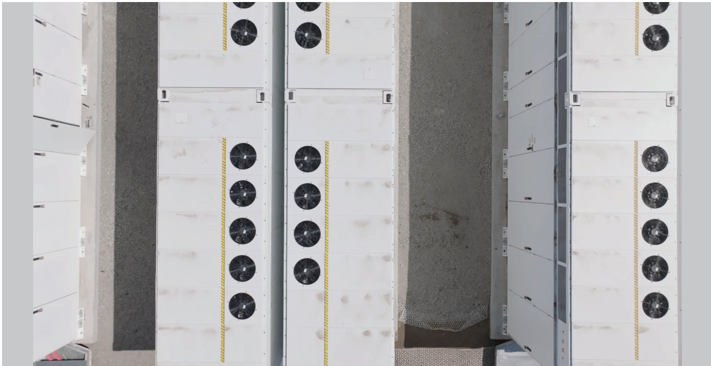
Superstition | Plus Power | Gilbert, AZ 90MW/360MWh BESS, Substation
