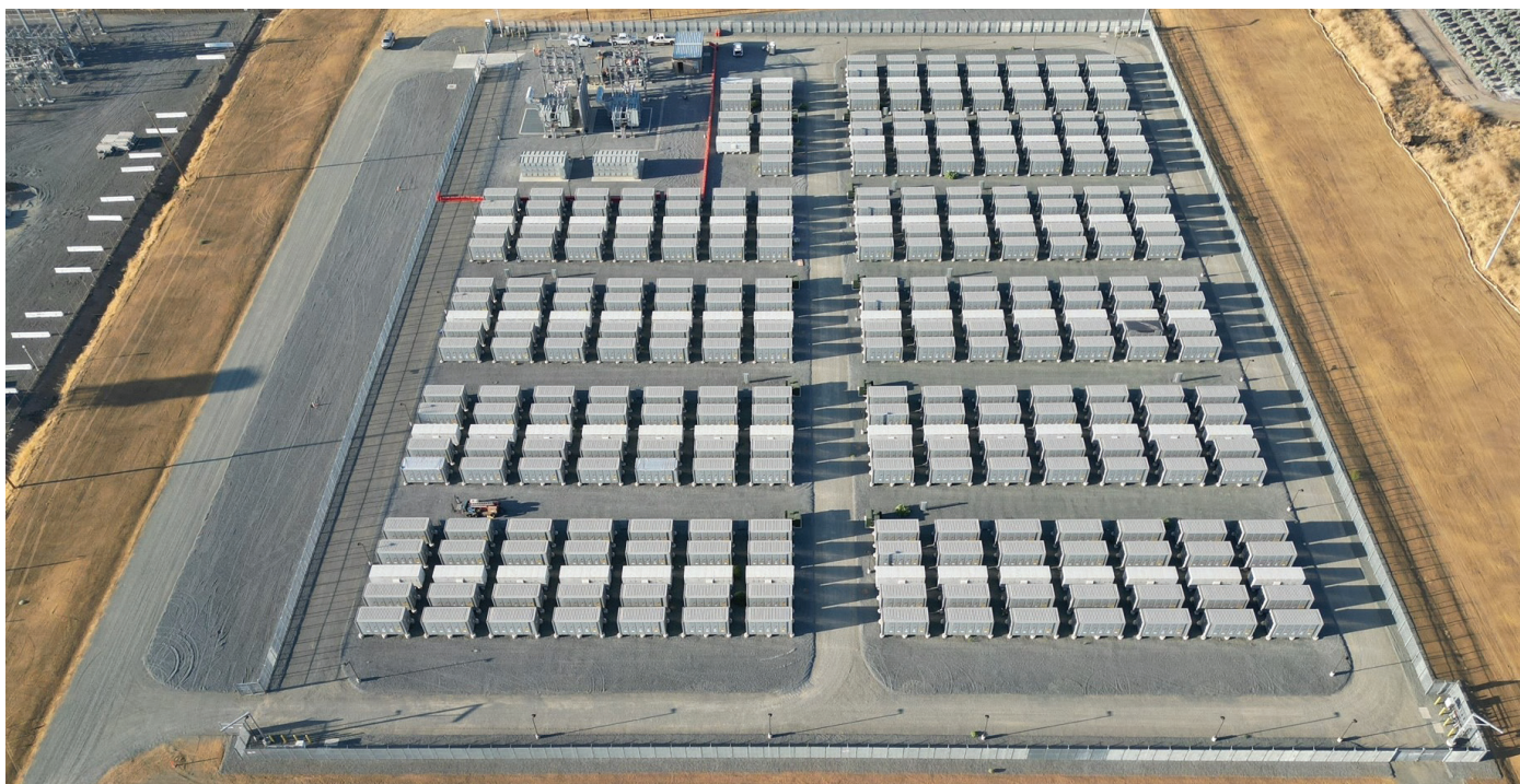
Southern California Energy Storage | Ameresco | Porterville, Rancho Cucamonga, and Long Beach, CA 537.5MW/2.15GWh (across 3 sites)
