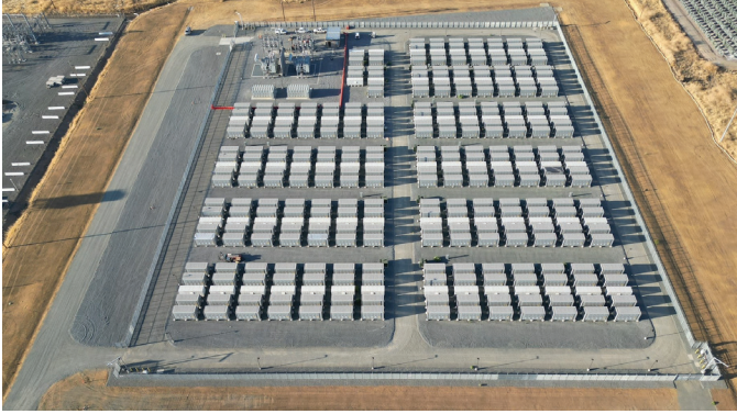
Southern California Energy Storage 537.5 MW/2.15 GWh across 3 sites BESS
