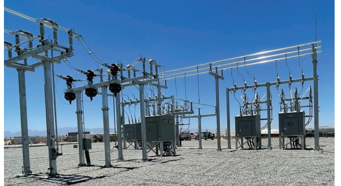
High Desert | Victorville, CA 230 kV substations US Fish and Wildlife and CA Department of Fish and Wildlife - Desert tortoise protection training Substation
