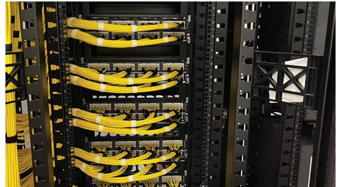
Hewlett Packard | Palo Alto, CA Design, project management, network cabling, audio/visual, security, wireless and rack/stack. Technology Infrastructure
