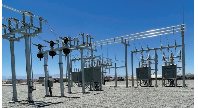
High Desert | Victorville, CA 230 kV substations US Fish and Wildlife and CA Department of Fish and Wildlife - Desert tortoise protection training Substation
