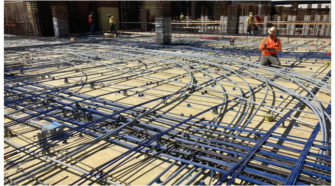
NBC Universal | Los Angeles, CA Building automation systems (BAS) low-voltage cabling Technology Infrastructure
