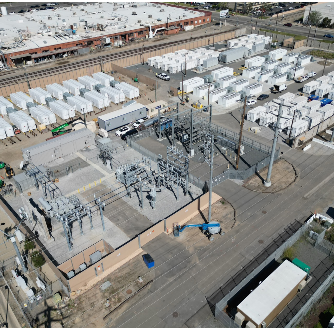
Santa Ana Energy Storage | Calpine California 40MW/160MWh BESS
