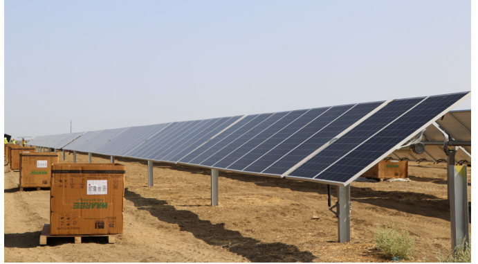
Aquamarine | Stratford, CA 250 MW solar, 1MW/2MWh BESS, 230kV Substation | BESS
