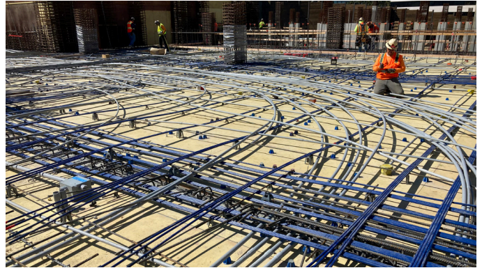
NBC Universal | Los Angeles, CA Building automation systems (BAS) low-voltage cabling Technology Infrastructure
