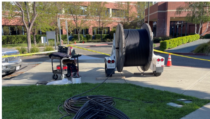
Stanford Tri-Valley Hospital | Pleasanton, CA Fiber optic network, backbone cabling, network cabling and upgrade to data center. Technology Infrastructure
