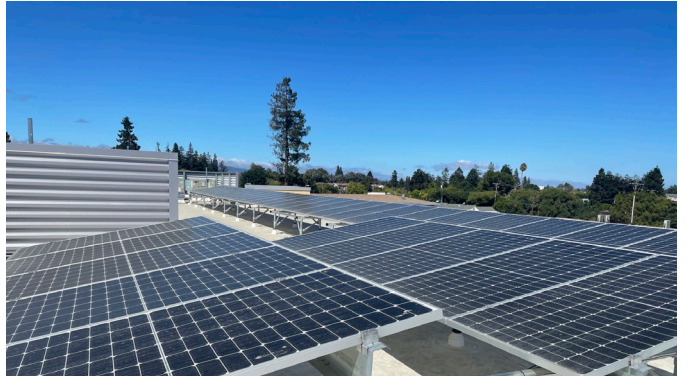
Mountain View Unified School District 1.6 MW canopy solar across 10 schools 12 EV charging stations EV Charging | Solar
