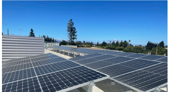
Mountain View Unified School District 1.6 MW canopy solar across 10 schools 12 EV charging stations EV Charging | Solar
